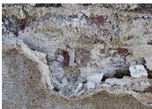
Typical damage through salt efflorescence.
